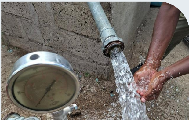
Oikos - Photovoltaic Water Pumping System in Longido District, Tanzania
